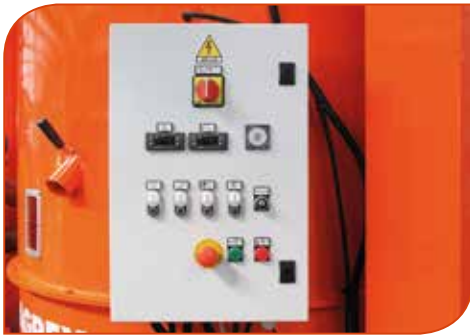
Electrical panel with integrated temperature sensors (air-product-safety) and timers
